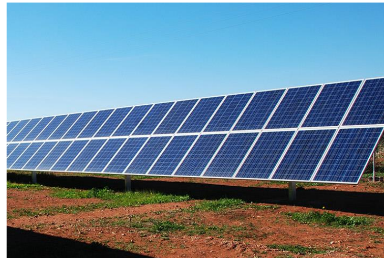
120 kWp – PV/Grid - Drip Agro-industry Morocco
